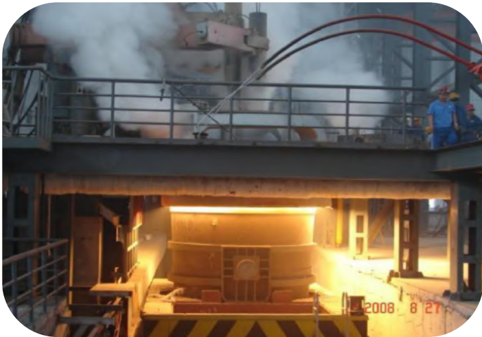
◆ 75t Ladle Refining Furnace
