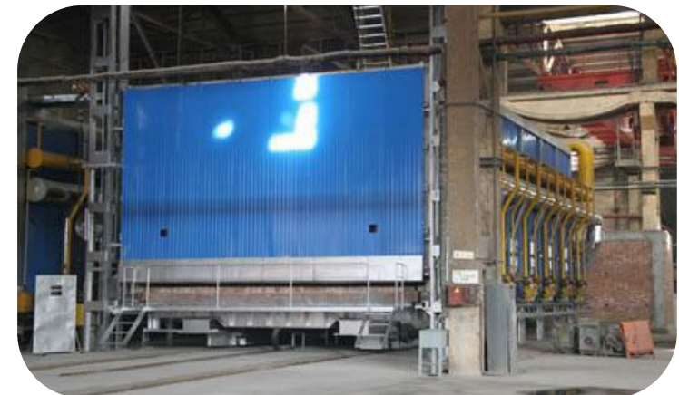
◆ 5X15m Heattreatment Furnace
