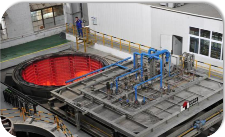
◆ \phi 5 \times 2.5 m Well Heattreatment Furnace
